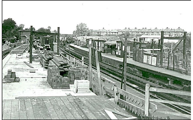
East Finchley looking north in the early states of the station's reconstruction and enlargement, showing the two main line tracks to the right and the future northbound Northern Line platform on the left. In the distance on the left can be seen the new LT signal cabin which appears to be structurally complete.
