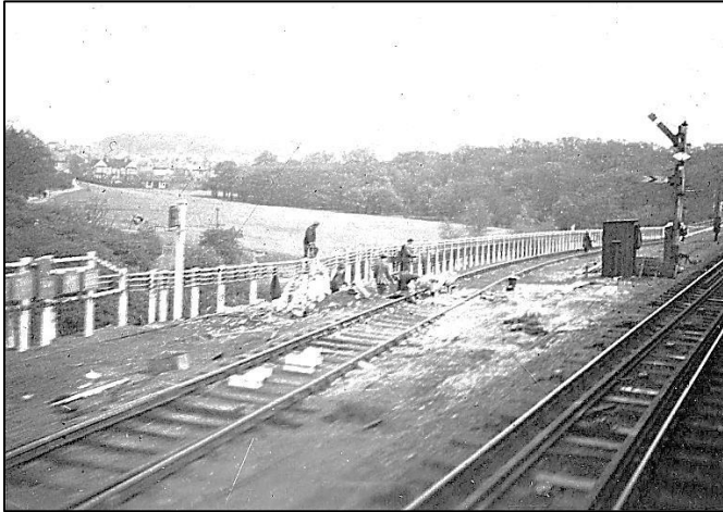
East Finchley looking south with work taking place on the extension of the Northern Line. New cable runs and a signal may be seen and track for the future southbound line is being laid. On the right is presumed to be the Up starting signal for main line trains.
