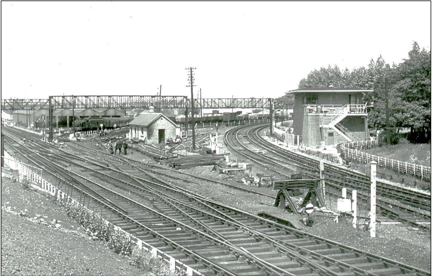
Above: Work progressing in 1939 at Park Junction in connection with the extension of the Northern Line. On the right is the new signal cabin at Park Junction, around which are the two tracks to and from Alexandra Palace, with some of the current rails laid. In the centre distance are what will become Highgate Wood Sidings for the Underground. To the left of the small brick building are the remains of Wellington Carriage Sidings for the LNER with the soon-to-be LT depot seen behind the steam train. The signalling is far from complete although some new signals and signal posts are in place.
